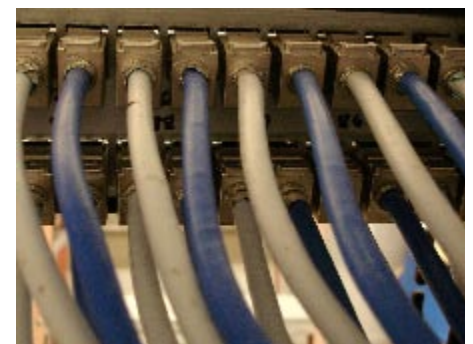
Over 2.1 million feet of 10 Gigabit shielded copper cable and 27,000 jacks are in Comcast Center.
