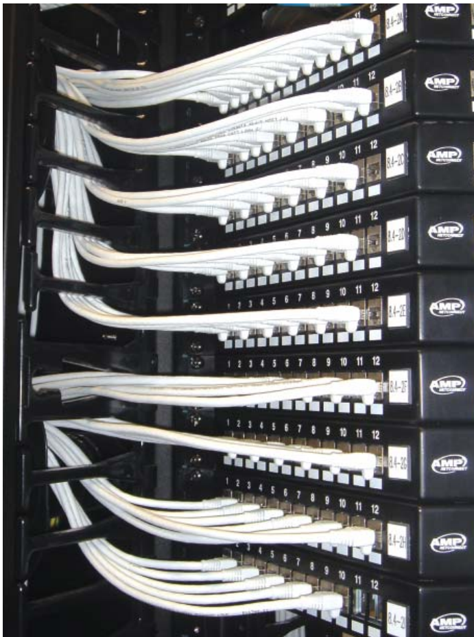
Above: Front view of AXA's high density cabinets utilising AMP NETCONNECT shielded patch panels, AMP-TWIST SL Jacks & Shielded patch cords.
