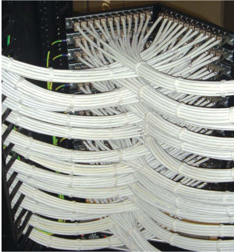
Above: Back view of AXA's high density cabinets utilising Class E A shielded cabling system.
