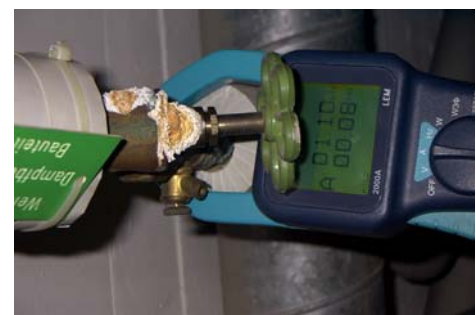
Corroded water pipe (GHMT AG)
