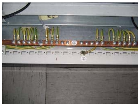
Fig 3: Terminal bar in a cabinet
